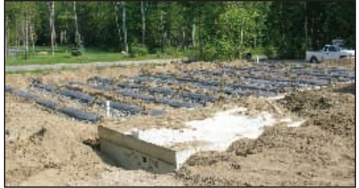
Septic tank and leaching bed.
